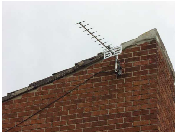
Figure 3: Damage at verge due to movement
