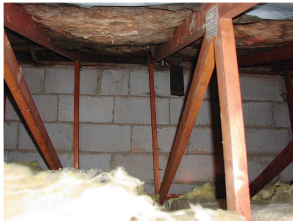
Figure 2: Further truss leaning
